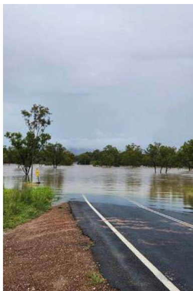
Multiple crossings have flooded.
