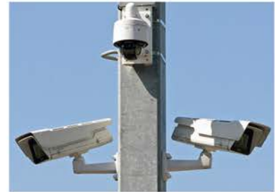
CCTV is on the increase.
